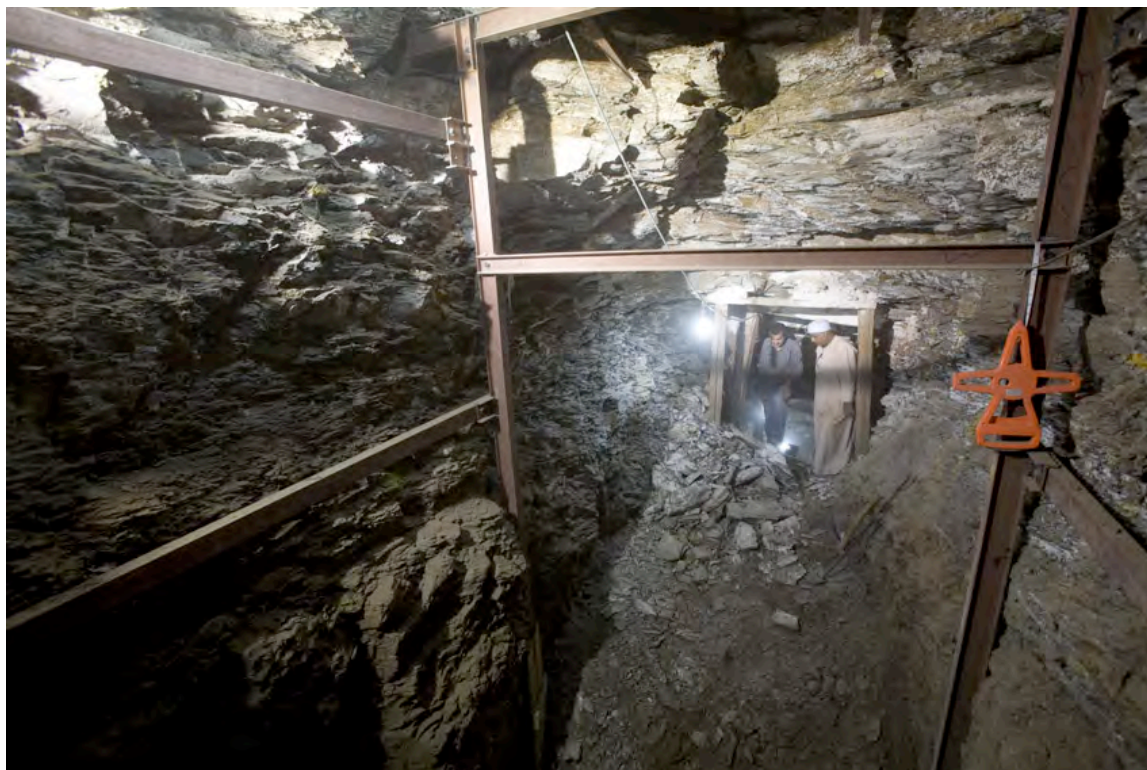
Steel reinforcement structure supporting the ceiling of the tunnel. (Photo by Sandro Vannini)
